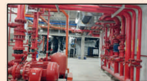
Fire Fighting System
